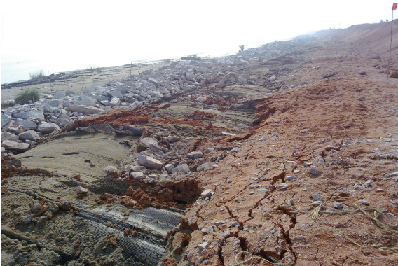
图2 小石坝变形和淤泥隆起 Fig. 2 Small rock dam deformation and silt uplift
