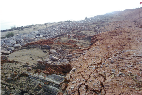
图2 小石坝变形和淤泥隆起 Fig. 2 Small rock dam deformation and silt uplift
