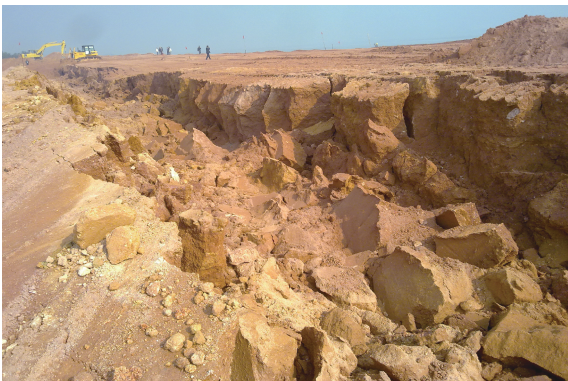
图1 护岸沿轴线方向开裂 Fig. 1 Cracking of revetment axis
